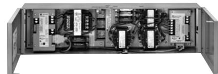
Voltage Module Interior View
